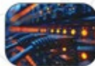
Networking Smart Racks
